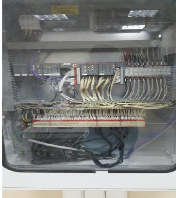
Figure.20 (Main PLC Board)
