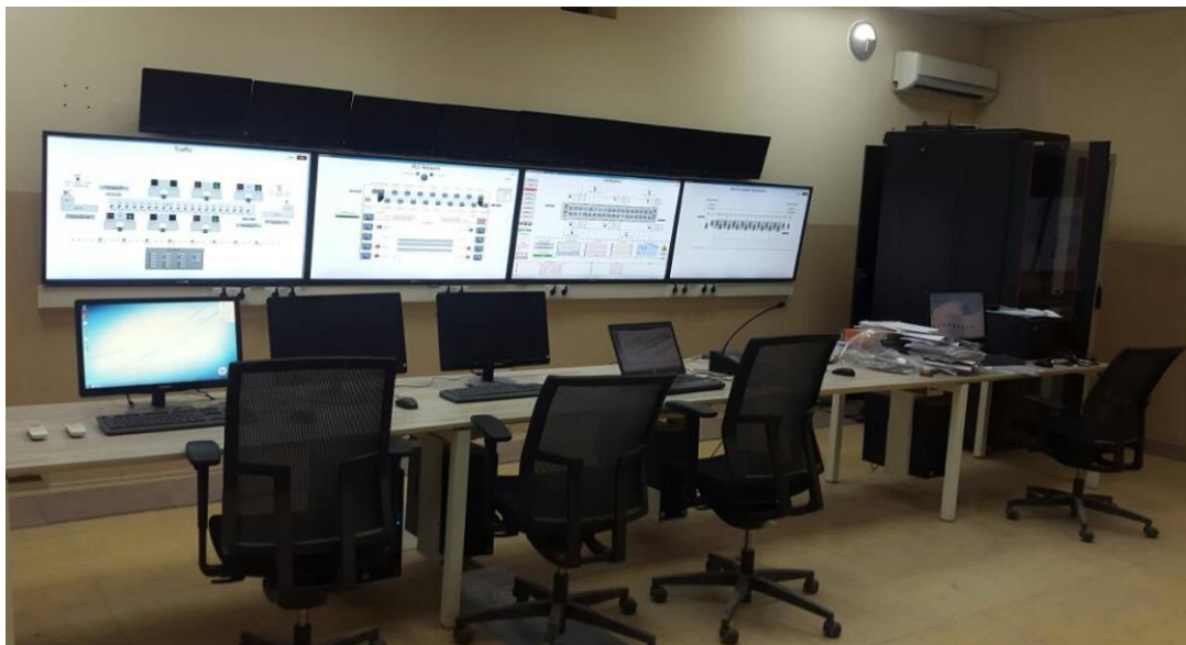
Figure.17 (Control Room of Peshraw Tunnel)
